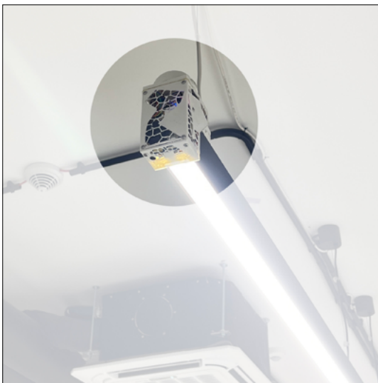
Fig. 9. The installed device.
