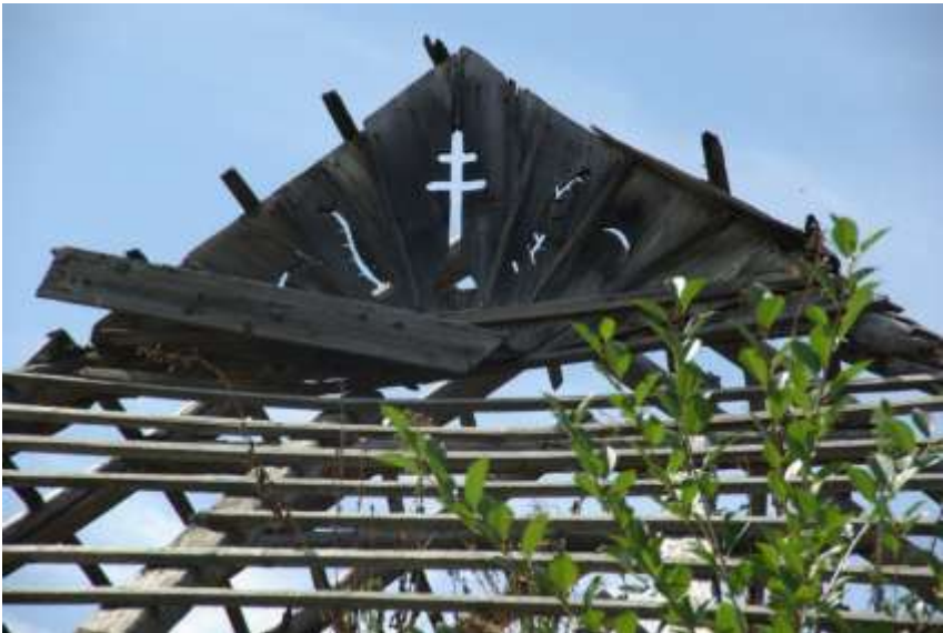
Figure 4. Open street view, only the pediment remains from the roof, the tree grew out of the wall
