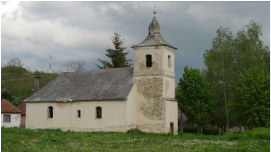
The dilapidated Reformed church without doors or windows and with a broken roof in Szakács.
