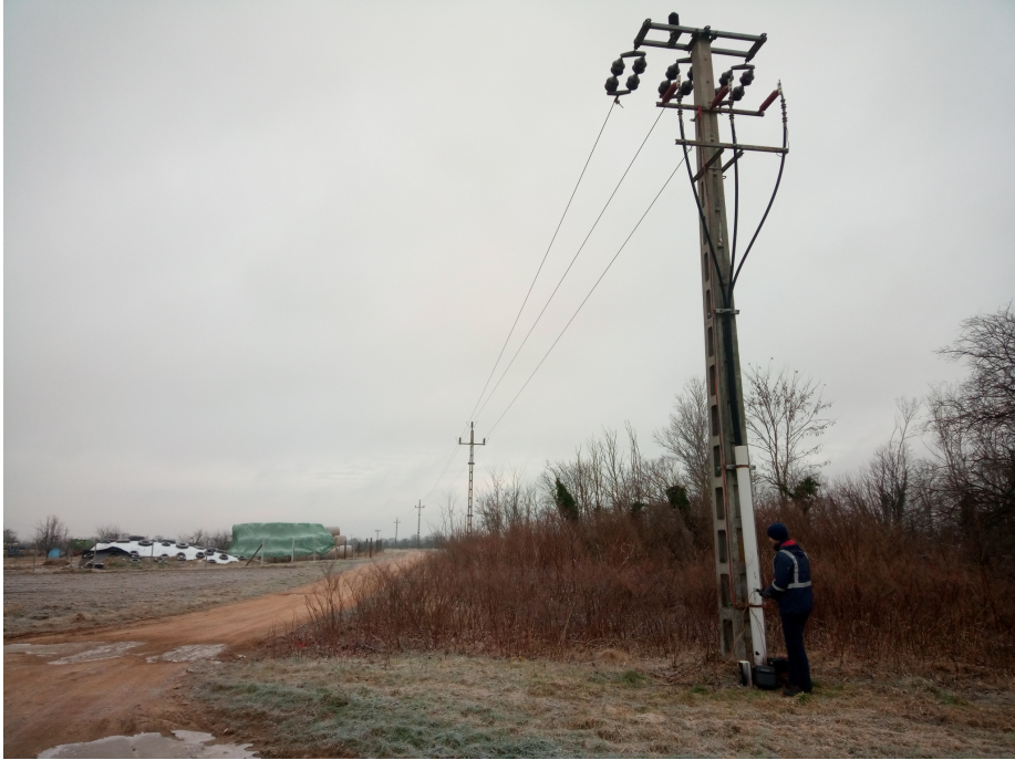
Fig. 4. Termination of the tested power line in Szakony. The three wires (phases) coming up from the ground and attached to the supporting pole are under power.
