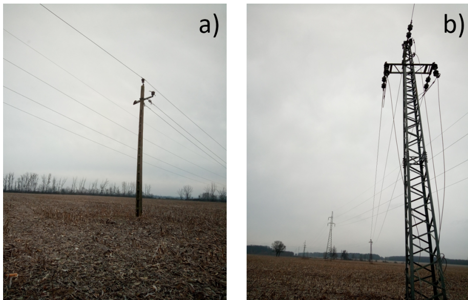
Fig. 3. Discontinuity (a) and loose grounding (b) of the tested unenergized power line. The other line is a high voltage transmission power line of 132 kV.
