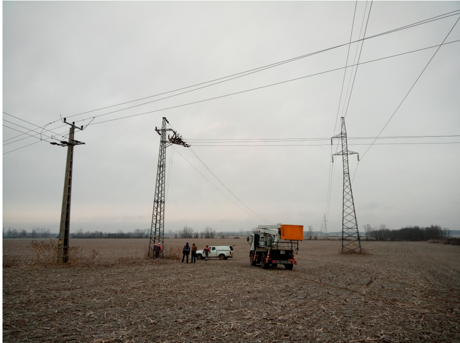
Fig. 2. Turning point of the tested power line, 2.2 km from its end in Szakony. The pole in the middle is equipped with a mechanical switch that allows breaking the continuity of the line.
