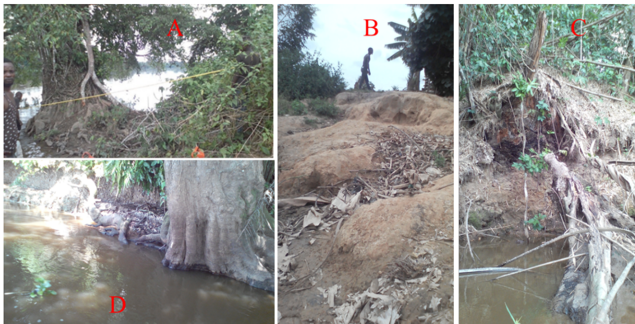
Figure 8. Mass movements, impacts and the role of trees in bank protection on the Kisangani–Belgica section. Result of erosion and landslides reported by residents on Mbie Island (A), erosion on Mbie Island (B), landslides on the right bank (C), landslides and erosion on the left bank (D)
