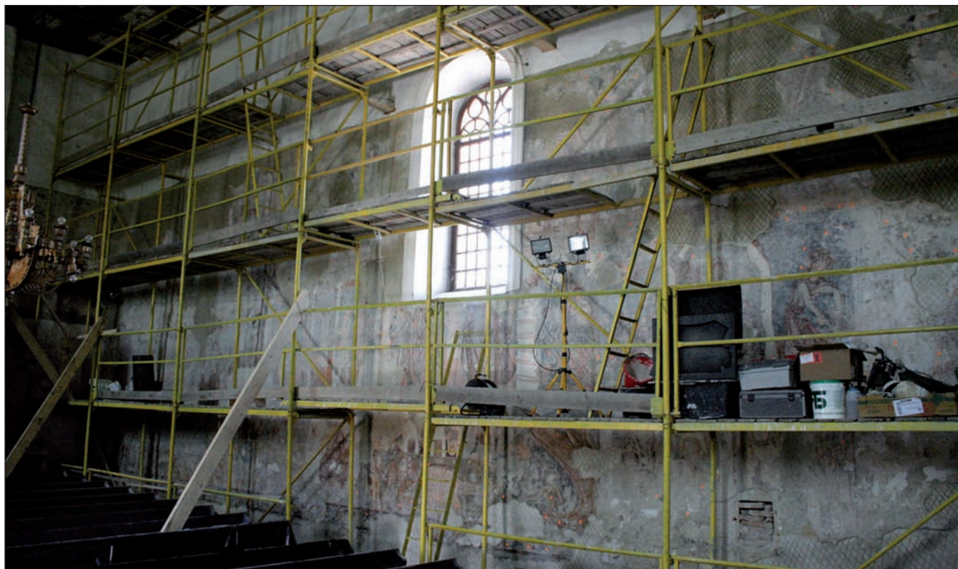
■ Photo 1. The northern wall of the Calvinist Church in Mugeni at the beginning of the conservation works
