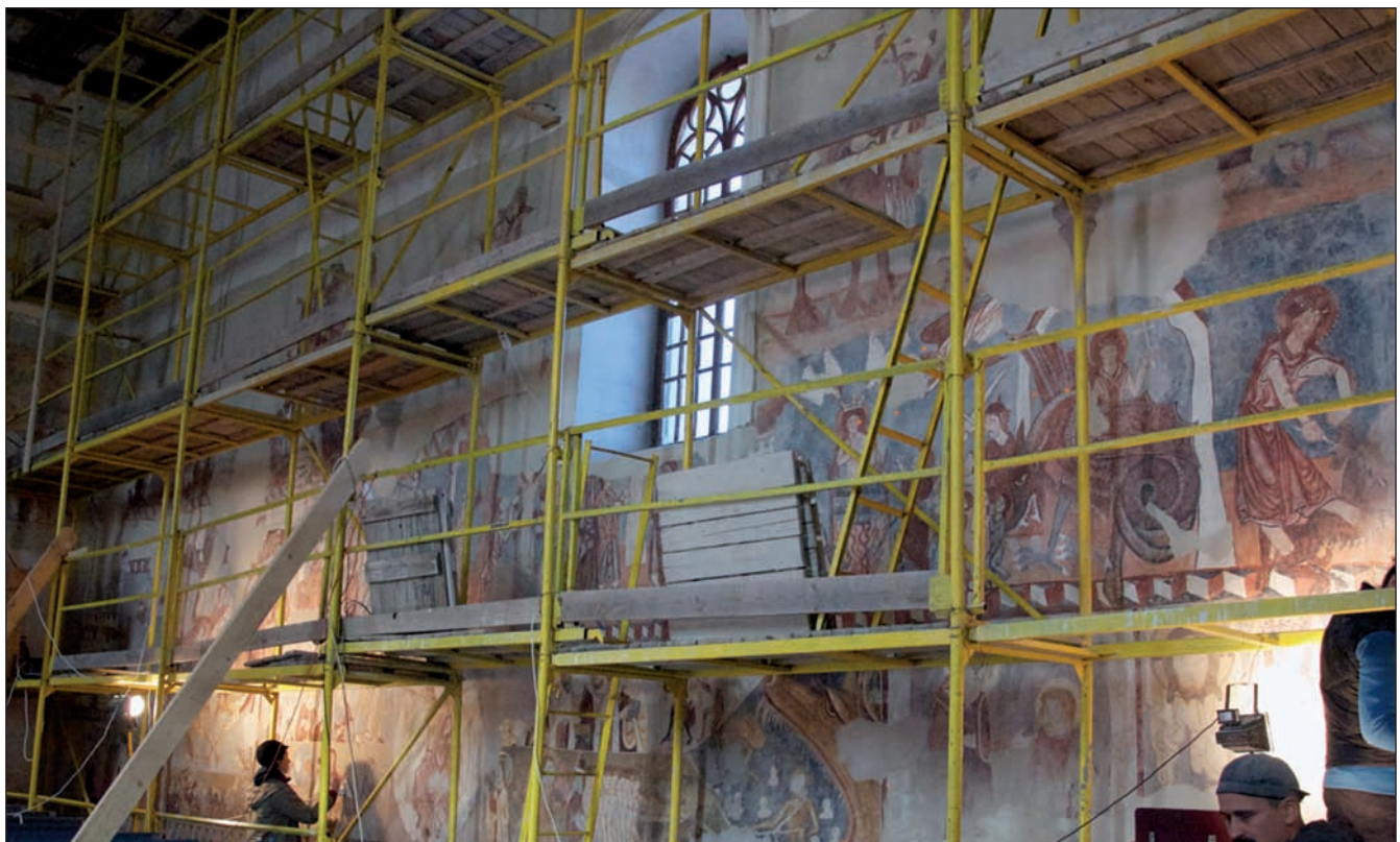
■ Photo 2. The northern wall of the Calvinist Church in Mugeni after preservation, during aesthetic restoration
