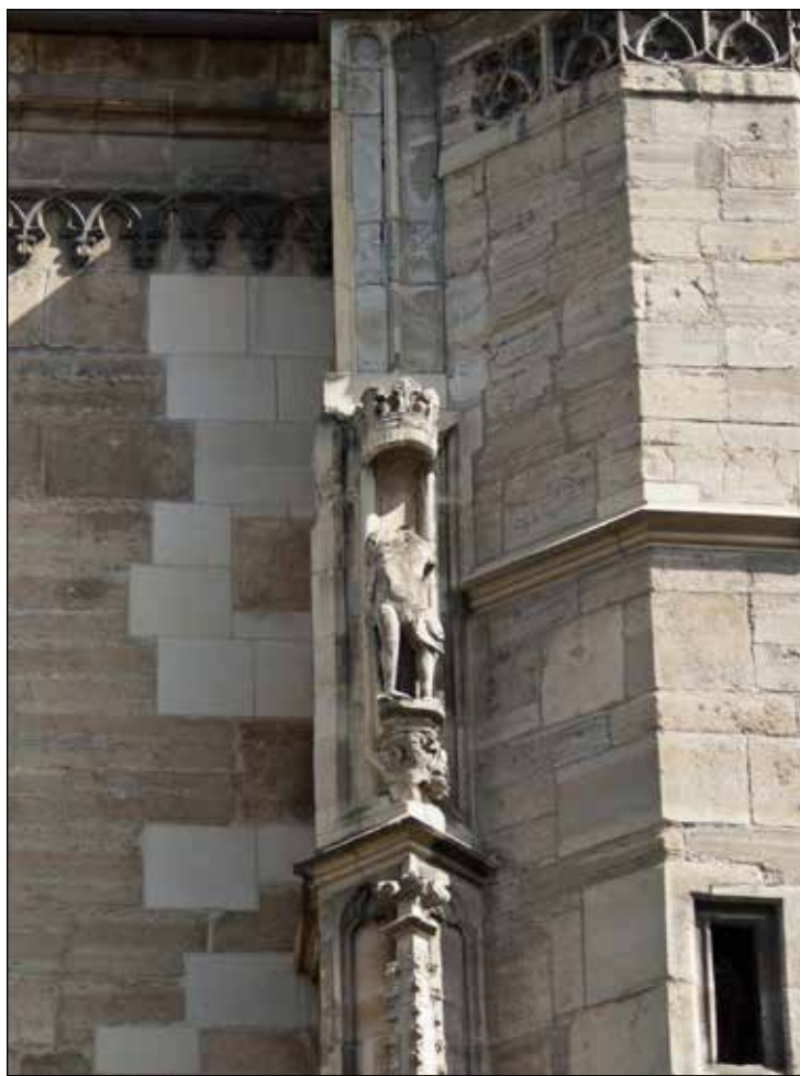
■ Photo 6. A corner on the southern elevation of St. Michael's Church with a clear difference between old and new stones © Anna KINDE
