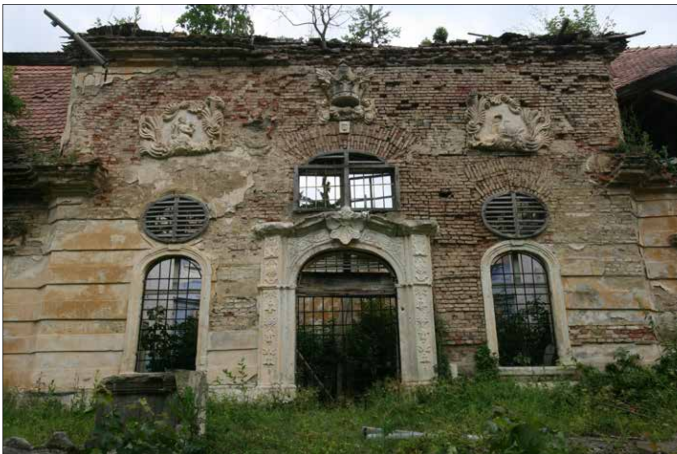
■ Foto 9. Rezalitul central al fațadei dinspre parc, 2015 © Zsolt KOVÁCS ■ Photo 9. Central projection of the elevation towards the park, 2015 © Zsolt KOVÁCS
