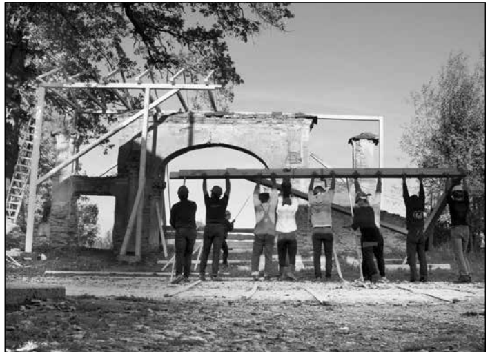
■ Photo 2. Building a timber protection for the Brâncovenesc-style gate from Sâmbăta de Jos (Braşov Co.), 2016 © MONUMENTUM Association
