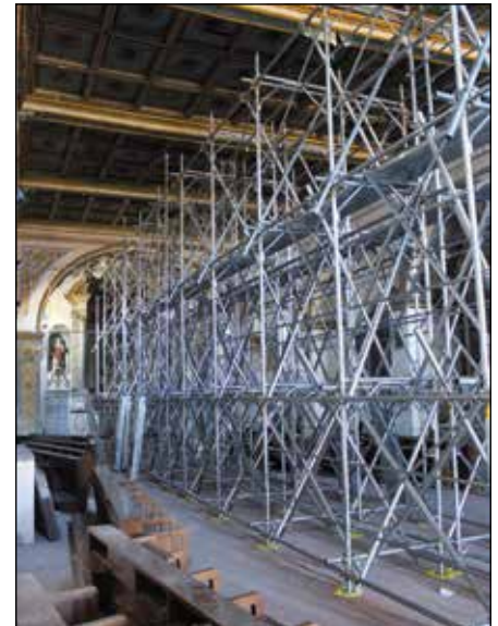
■ Photo 6. Monteleone di Spoleto, S. Nicola. Temporary works installed by the author (2017)
