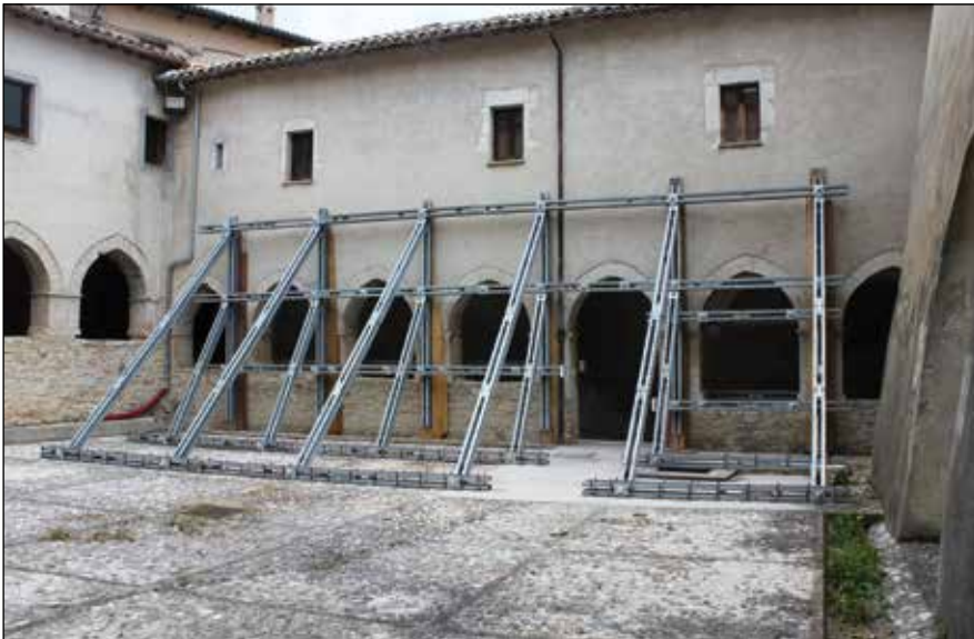
■ Photo 5. Monteleone di Spoleto, S. Francesco, cloister. Temporary works installed by the author (2017)
