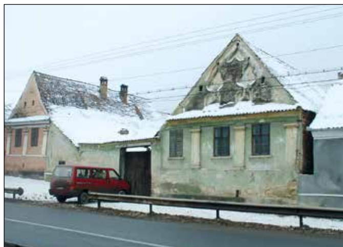
■ Foto 3. Saschiz, nr. 30. Fotografie de monitorizare © INP, 2004 ■ Photo 3. House No. 30, Saschiz. Monitoring photograph © INP, 2004
