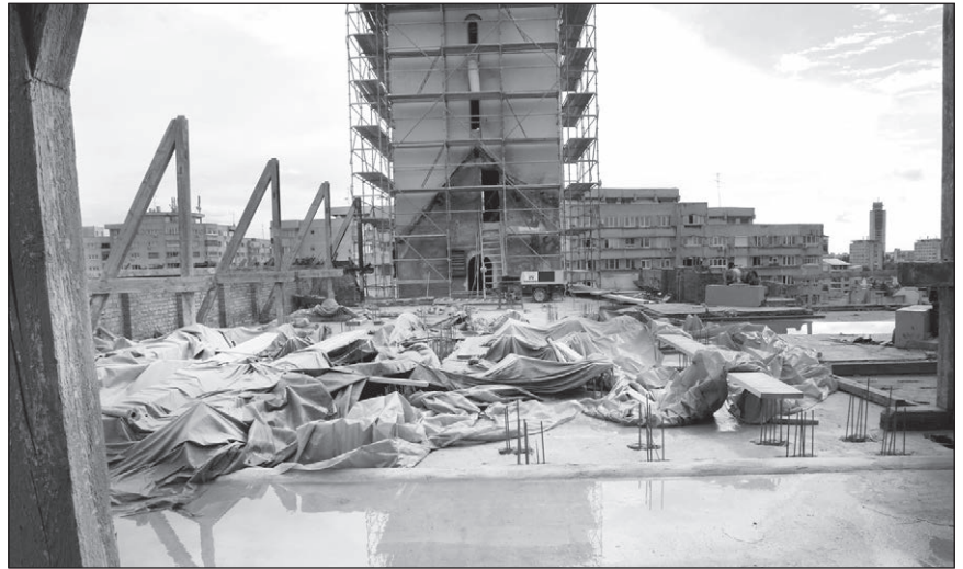
■ Photo 1. The Town Hall of the 1 st District in Bucharest – the remains of the roof structure after the 2009 fire
