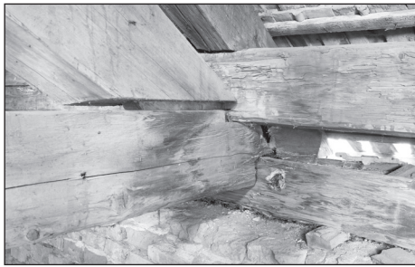
■ Foto 6. Detaliu nod curent pană - căprior. © Adrian TUDOREANU ■ Photo 6. Detail of intermediary purlin – common rafter joint. © Adrian TUDOREANU
