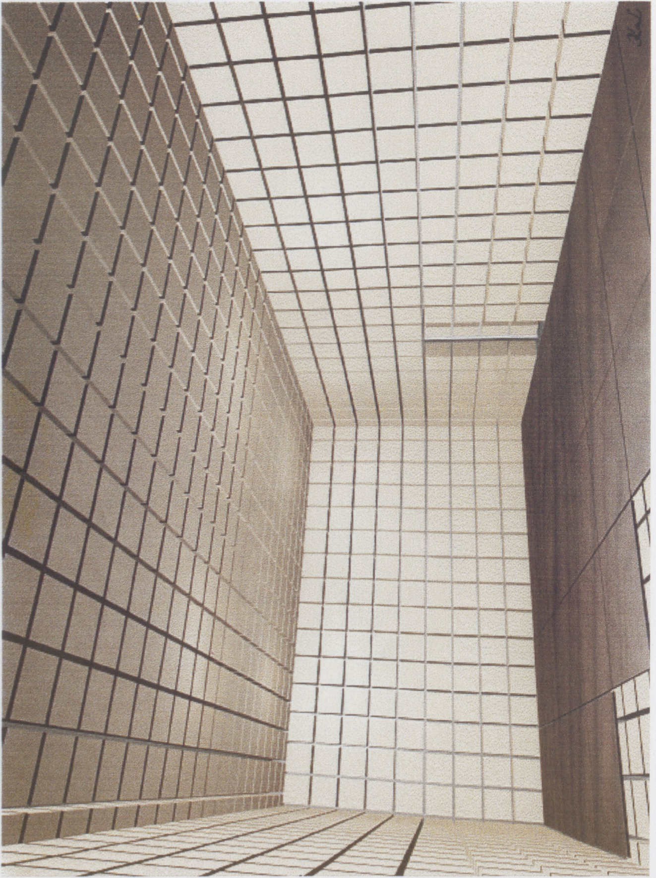
Fig. 5. Anechoic chamber using our absorbers (suggested for EMC tests in the 80-1000 MHz frequency band)
