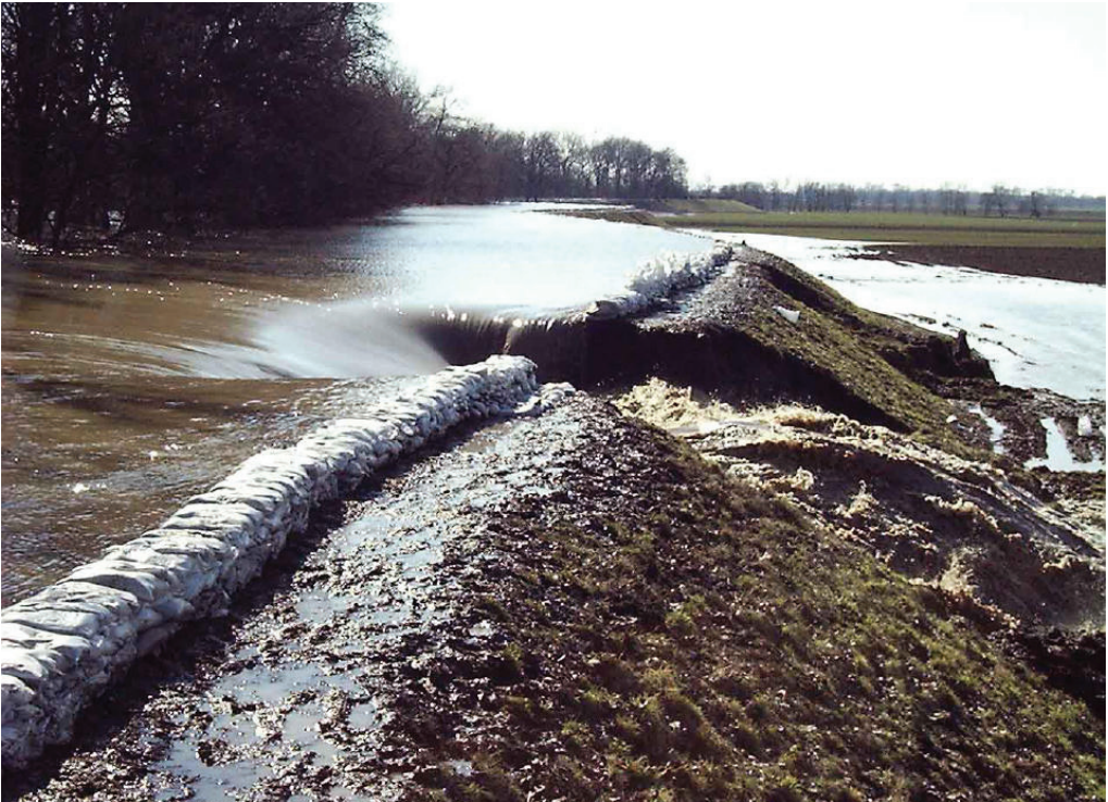
PICTURE 1 ♦ Dam break in Tarpa. (Photo: www.tarpa.eu )
