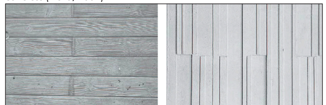
Fig. 2: The impression of the formwork structure on the surface of the concrete (Doka, 2009)
