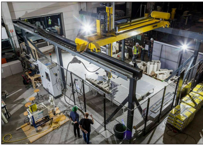
Fig. 18: Concrete elements 3D printing (3DCP) at Eindhoven University of Technology (Project Milestone, 2019)
