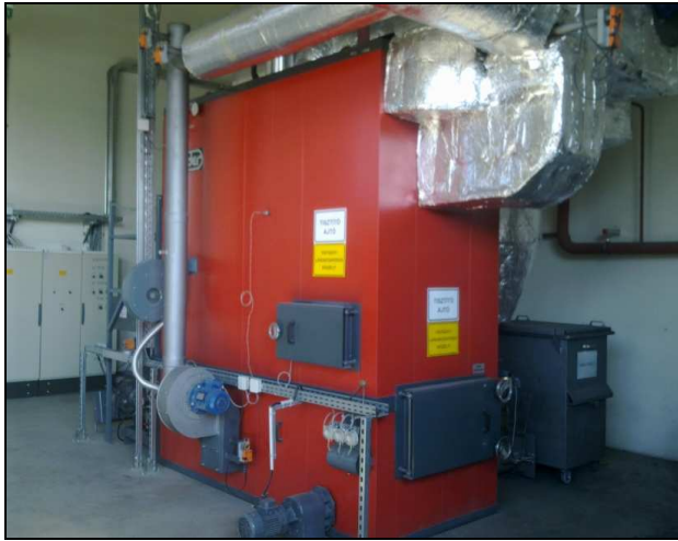
Figure 2. Photo of the examined boiler (semi-plant scale experiment)
