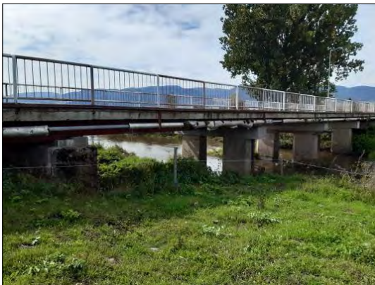
Fig. 4. The road bridge built over the widened riverbed on the site of the old arched bridge.
