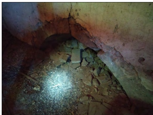
Figure 1. The remains of the walled-up Gothic lancet windows located in the attic.
