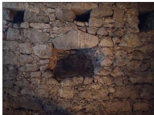
Figure 2. The three smaller holes and one bigger hole with a stone functioning as a lintel in the attic's gable wall.
