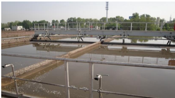
Figure 1. Rectangular settling basin
