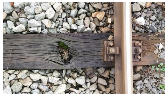
Figure 6. Defect of a wooden sleeper
