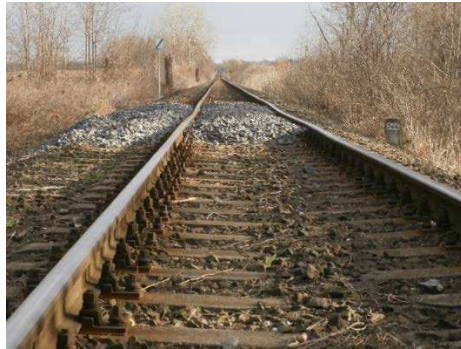
Figure 12. Local substructure failure [32]
