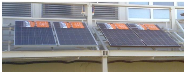
Figure 7. Shading of PV modules
