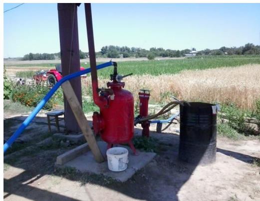
Figure 3. Water cleaning and additional fertilizing system
