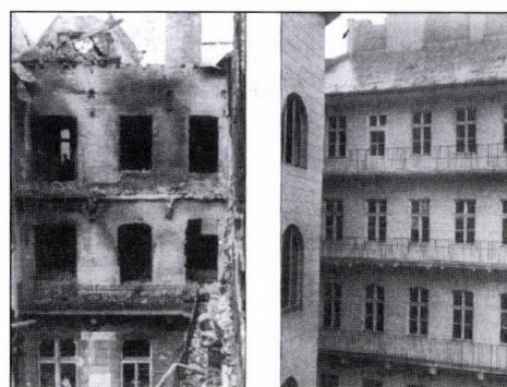
The building of the Department of Zoology before and after the reconstruction
