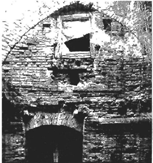
Fig. 3. The south-eastern interior corner of the basilica. Superimposing of the different periods in the openings in the southern exterior wall.
