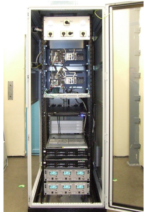
Figure 2: Cabinet of ANEREM components near to the MCR
