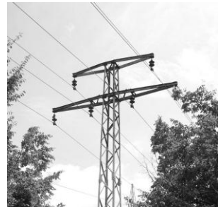
Type 3. Metal structure with insulators fixed downwards and 6 lines
