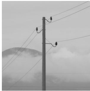
Type 2. Concrete pole with insulators fixed upwards and 3 lines
