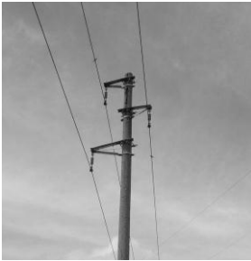
Type 4. Concrete pole with insulators fixed downwards and 3 lines
