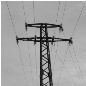
Type 1''. Metal structure with jumper wires and 6 lines
