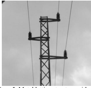
Type 5. Metal lattice structure with insulators fixed upwards and 3 lines
