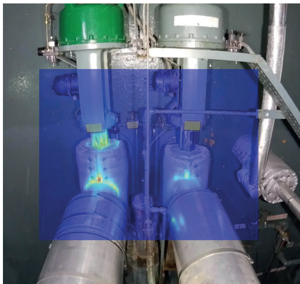
Figure 6. Thermal camera image showing a pipeline leak [11]
