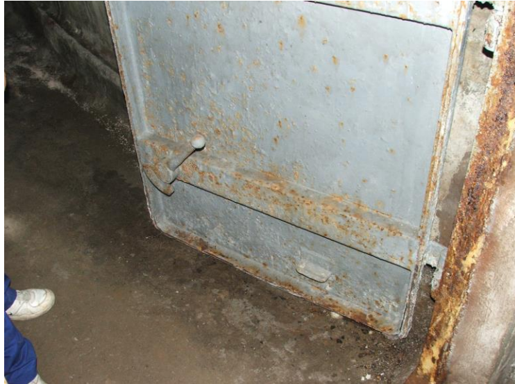
Figure 13: Protective door corroded due to the absence of maintenance in the KAGRA facility 21
