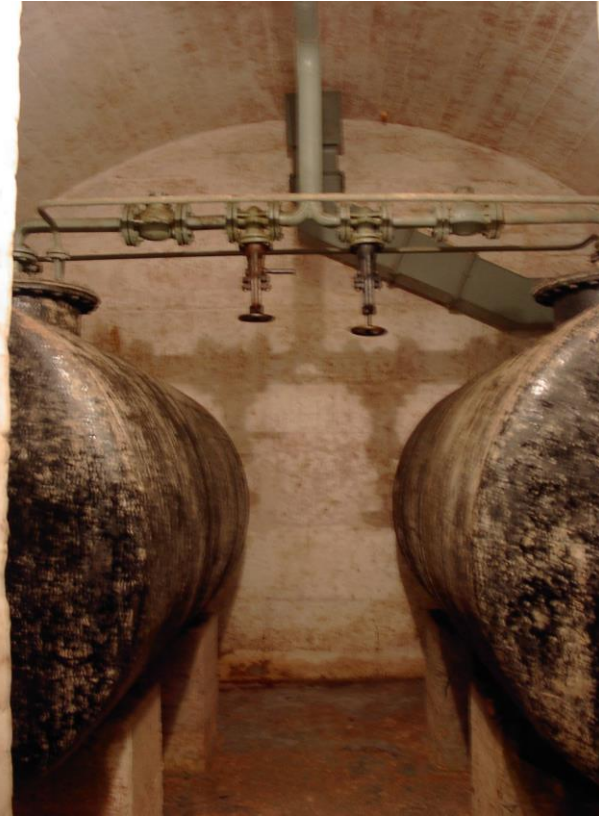
Figure 17: Fuel tanks in the Hospital in the Rock in Budapest 27
