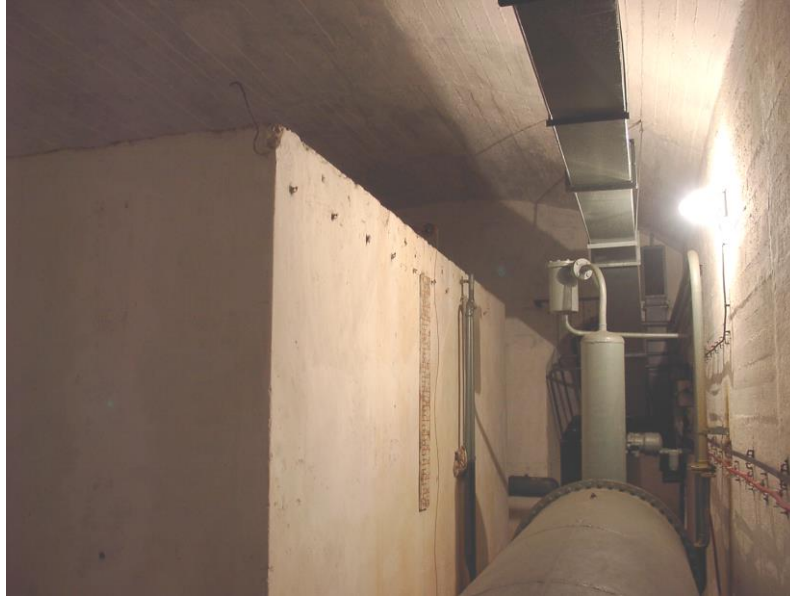
Figure 16: Reinforced concrete drinking water container in the Hospital in the Rock in Budapest 26
