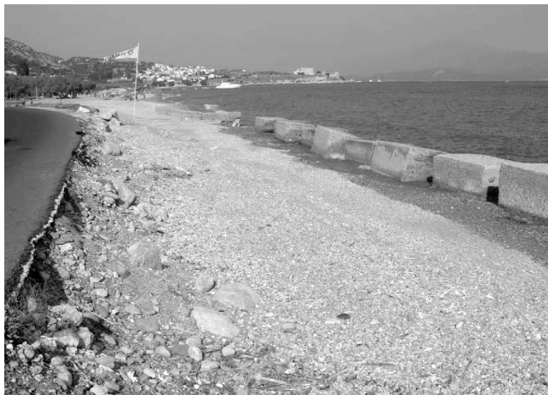
Figure 9. Coastal erosion causes problems to the southern part of the island as well.
