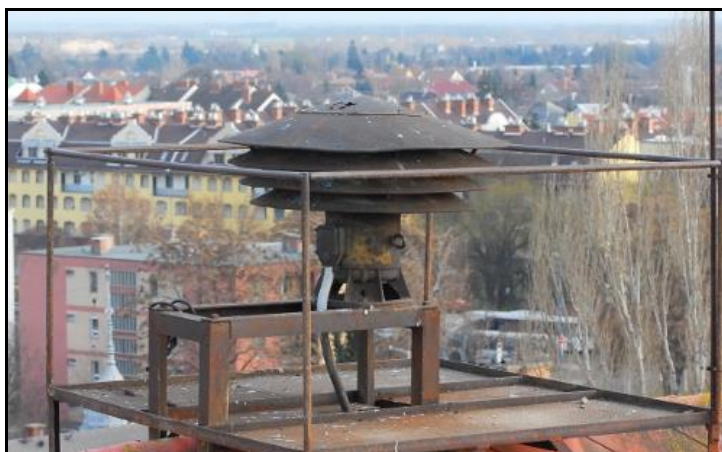
Figure 4: Szentes City's main siren which was sounded after 23 years (Performance 5 kW)
