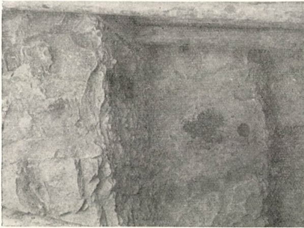
Fig. 6. Stepped foundation plane in the hard, bedded Buda marl at depth from 8 to 10 m below terrain surface
