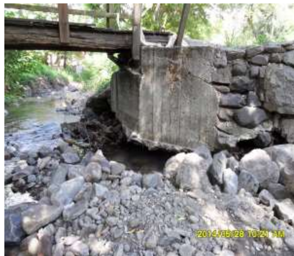
Further damage (photo taken by the author)
