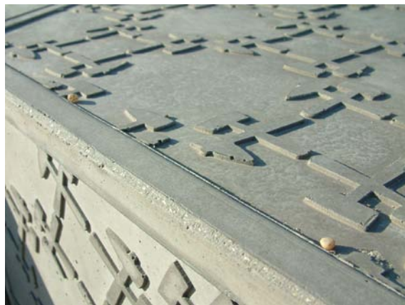
Photo 4: The Tettye-park furnitures' roughly chamfered edges
