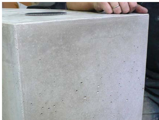
Photo 2: The surface of a slightly airholed concrete bench after being chamfered
