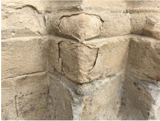
Fig. 9.: Flaking of molasse sandstone due to thermal/hygric dilatation and/or freeze-thaw cycles on the footing of the Parish church in Schöngrabern, Lower Austria (image courtesy J. Nimmrichter)
