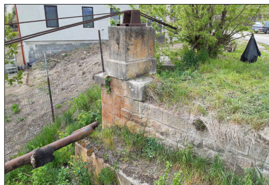
Figure 2. Ahe current state of the abutment
