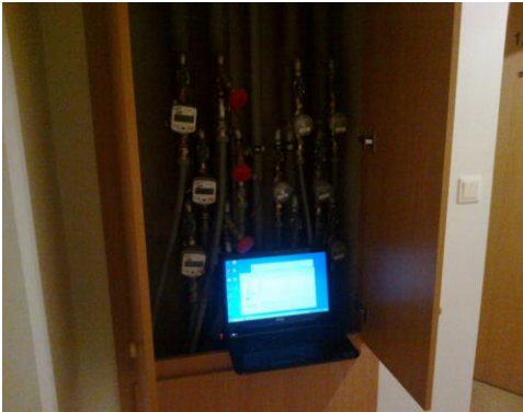
Figure 3. Receiver in water and heating meter cabinet
