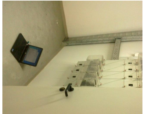
Figure 4. Receiver in electric meter room
