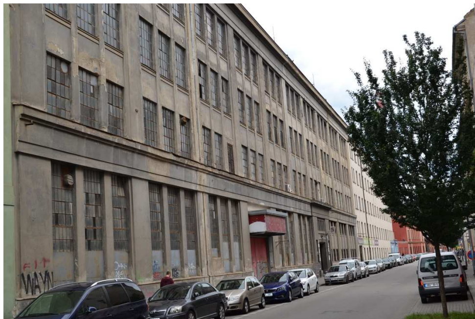
Figure 2 An example of the neglected and the dilapidated building of industrial brownfield at Špitálka Street in Brno
