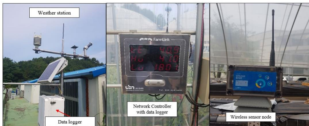
Figure 2. Images of local weather station, network controller with the data logger, wireless sensor nodes used in the experimental site
