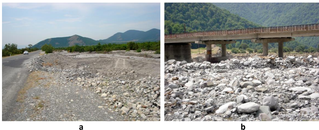
Figure 6. a The section of the highway Sheki-Oguz, blurred as a result of mudflow on the river Kishchay. b Bridge damaged by the mudflow in the valley of the Chukhadurmaz river (tributary of the Kishchay river)
