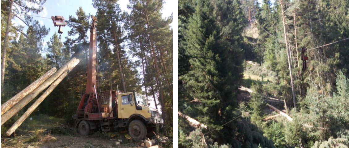
Figure 1. Urus MIII cable crane
