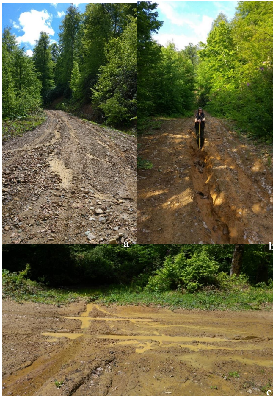
Figure 3. Unpaved road segment samples. a Sediment transport along the rills that form on the road segment. b Highly eroded road surface. c Erosion on the node where two road segments intersect
