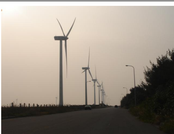
Figure 30. The first turbine is No. 21
