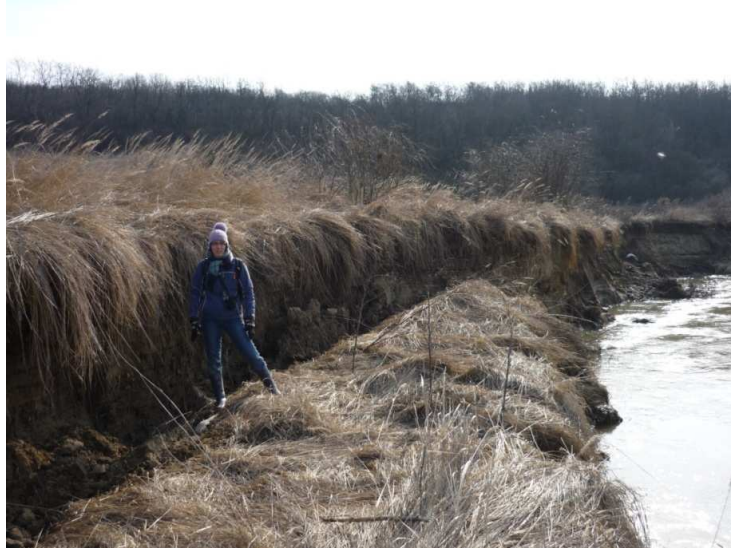
Picture 1. Block collapses along the river bank which covered by natural vegetation
