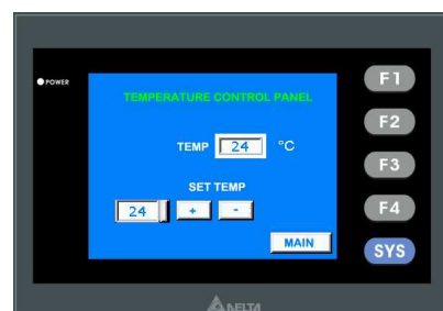
Figure 12 Temperature control panel
