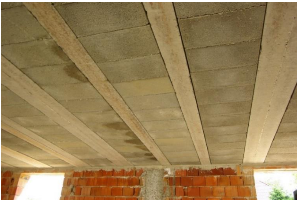
Figure 5: Incorrect slab design (Made by: Péter Tóth)
