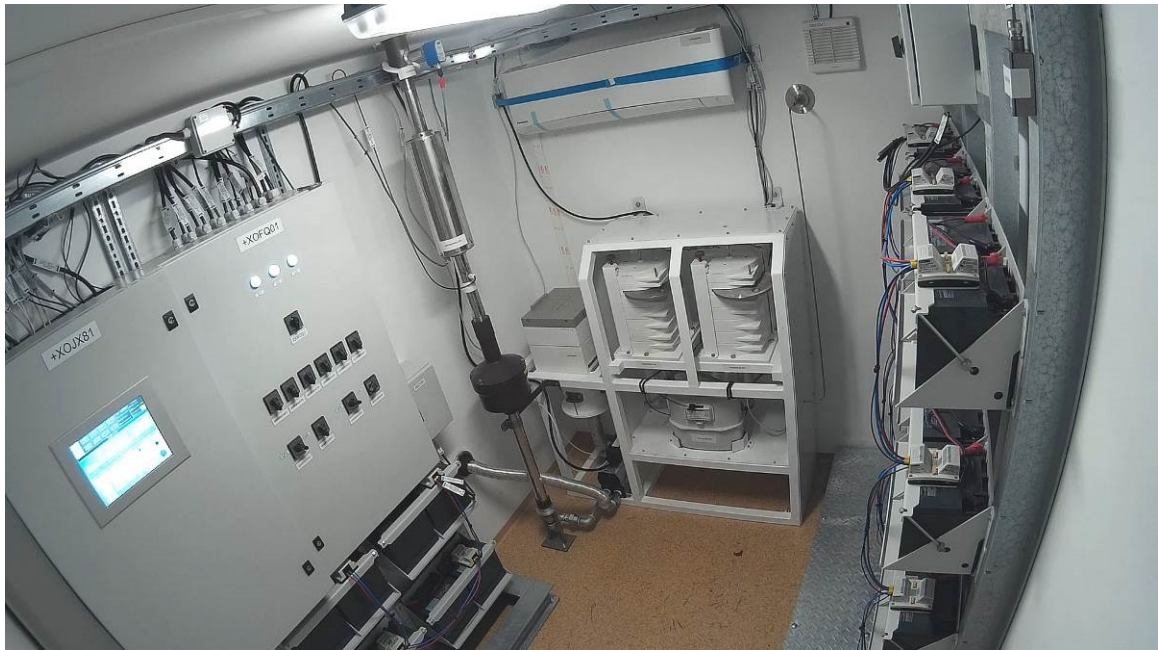
Figure 2: One of the camera views inside the container during earthquake resistance test
