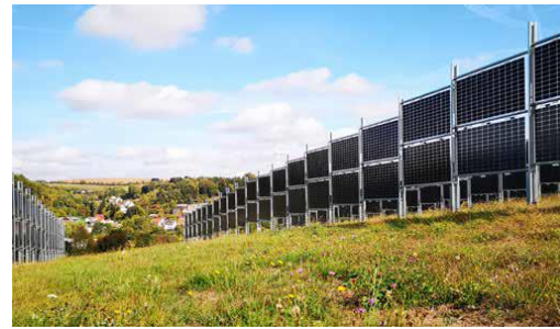
Figure 2. Bifacial modules installed vertically, Donaueschingen-Germany. @Next2Sun GmbH
