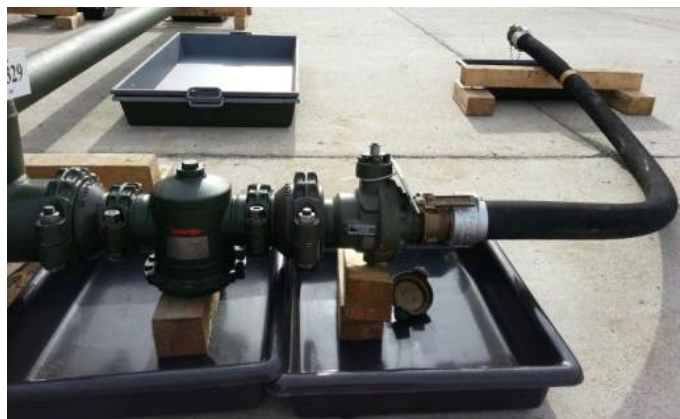
8. Figure. Filling Point with Flow Limiter (Photo made by the author)
