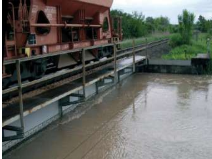
Figure 6. The water of Szuha Stream reached the bridge structure on line 81 [8]
