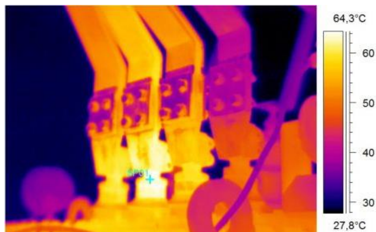
Fig4. Un-Torqued connection around the ceramic insulator. T phase connector is about 70 C. [18]
