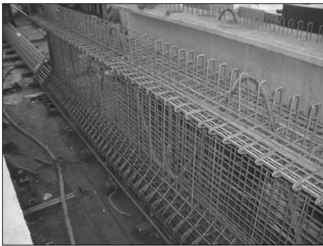
Fig. 6: A part of the reinforcement cage with two lifting hooks at the FI-150 beam end
