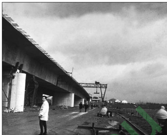
Fig. 12: Construction of the bridge across the Waal River, the flood area structure. (In the figure D. Dalmy, member of the Hungarian delegation, today manager of Pannon Freyssinet Ltd. and member of the Palotás László award board of trustees of Hungarian Group of fib )
